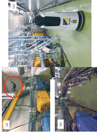
Fig. 2. a) Drone test in the MR tunnel. b) Video from the drone. c) Robot demo in the MR tunnel.
