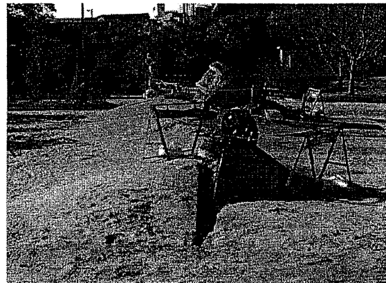
Photo 2 Uplift of underground water tank (Chiba Pref.) 7) .
