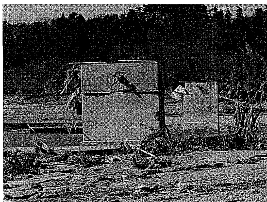
Photo 3 Damage to water pipe bridge (Miyagi Pref.).
