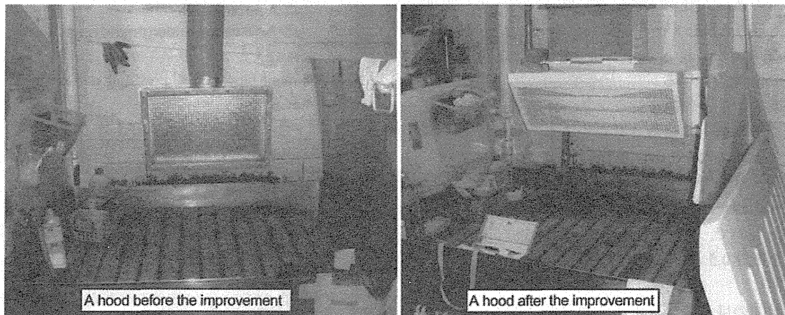
Fig. 6. A hood of local exhaust ventilation system in the washing space.
