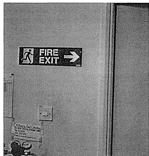
Fig. 16. Fire exit sign
