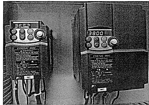
Fig. 5. Inverters I and II
