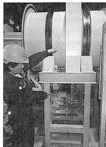
A guard was made from waste metal materials (= low cost) and attached to the moving part of a machine.
