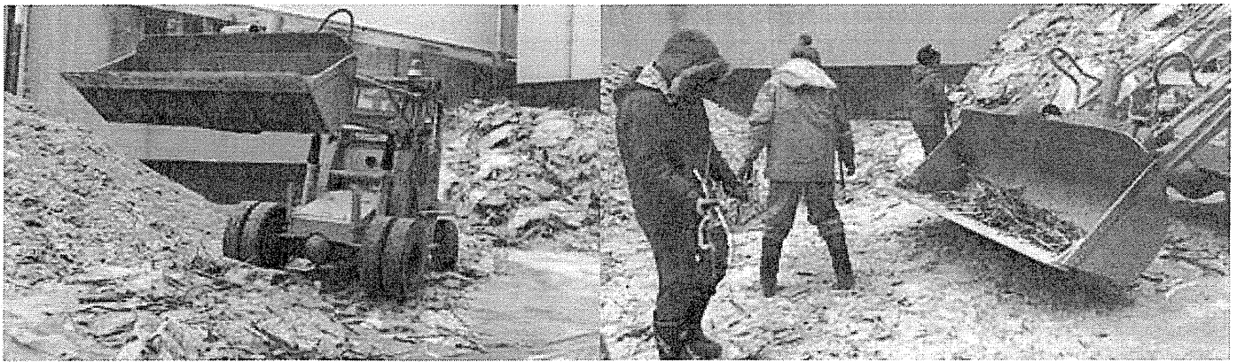
Work improvements in the preparatory process at the glass recycling factory. (Left) A heavy machine crushes waste glasses. (Right) Workers pick up metal frames.
