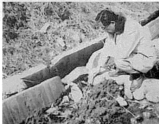
Figure 78. Examination of a damaged canal in 1980 in Tamaho town.
