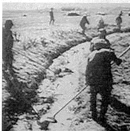
Figure 48. A long-arm dipper was used to spread the preparation on the wall of the canal.
