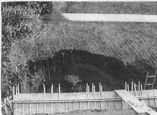
Fig. 6 Accident site at frame dismantling work
