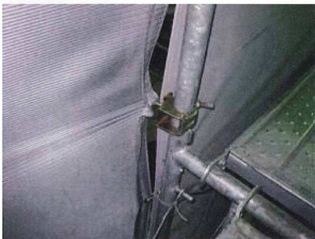
Photo 4. The plastic sheets bound to the pipe of the scaffolds with a special coupler.
