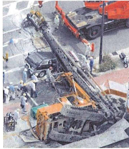
FIG.1. Overturning of a drill rig in construction site.
