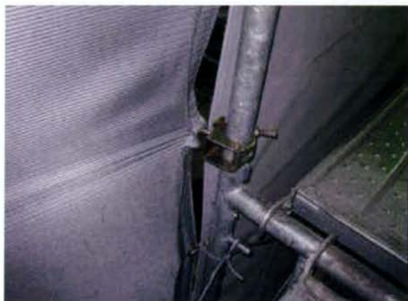
Photo 2. The plastic sheets bound to the pipe of the scaffolds by exclusive coupler
