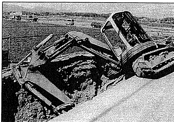
Photograph 1. Ground collapse during trench excavation
