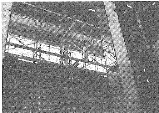
Figure 2 View of the experiment: The test being carried out is with a 240 mm-wide footing board.
